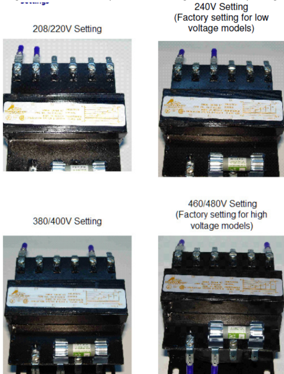
Figure 6 – M700 Helium Compressor Control Voltage Transformer Tap Settings
